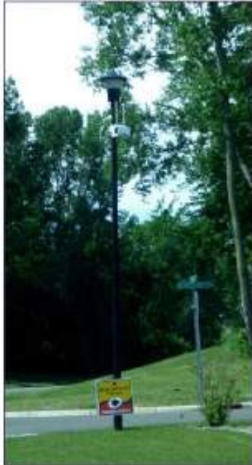
The Tropos 5110 outdoor MetroMesh router.
