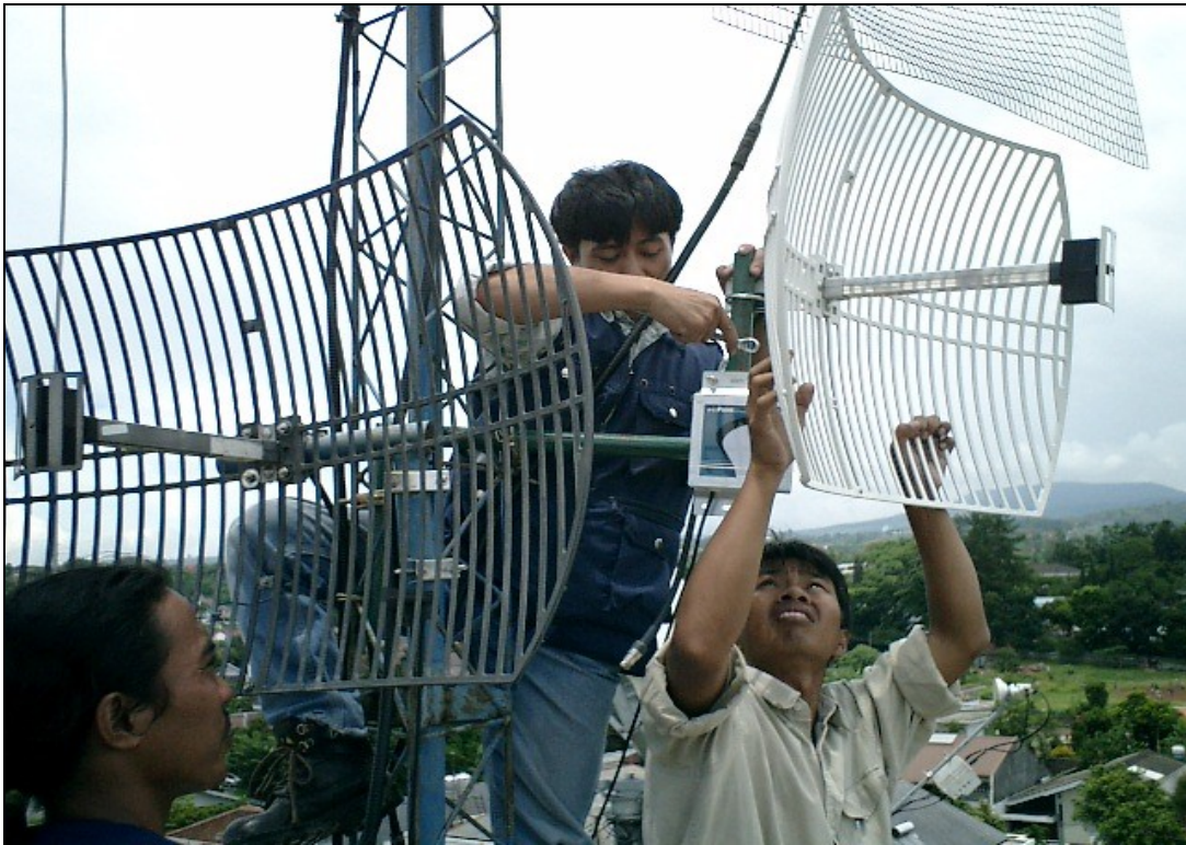
Image 22: Access Point installation in the wireless “hub”
