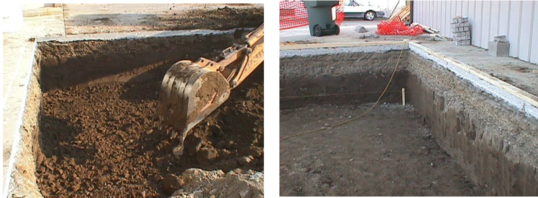
Image 5: a) Digging the hole for the base with a backhoe b) The hole is finished with straight and even edges.
